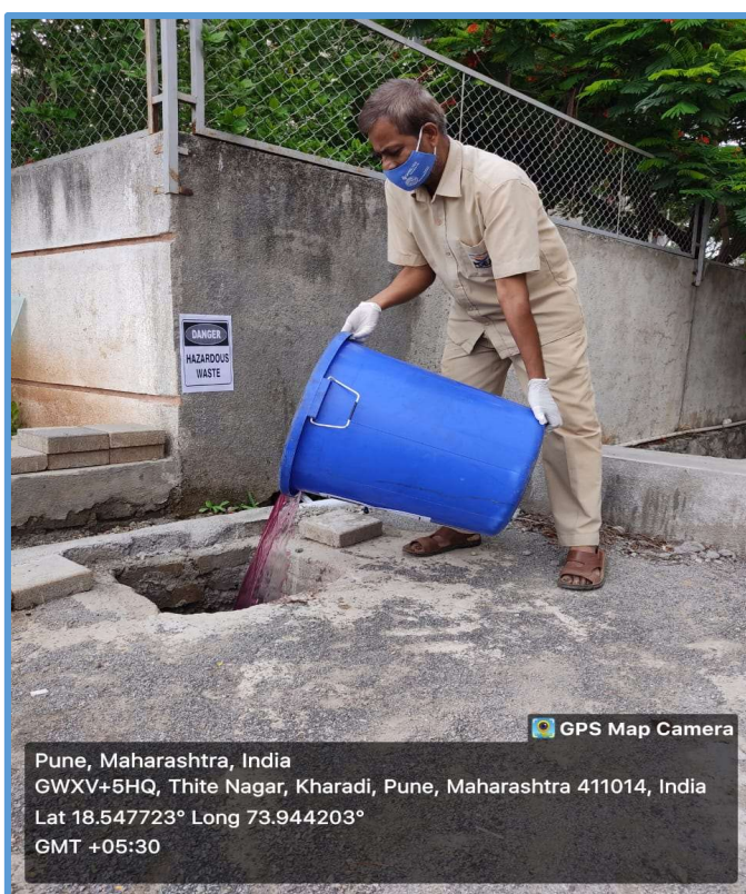
Soak Pit for Hazardous Liquid
